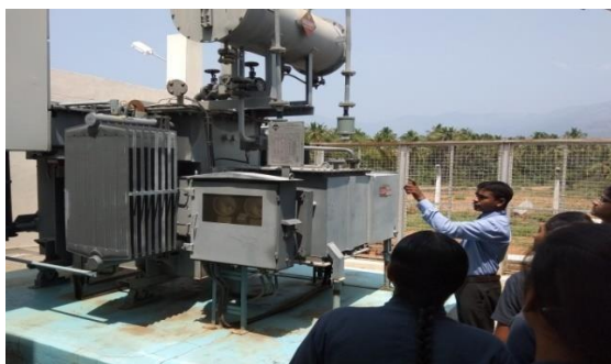
Students at Field Visit – “RIT Power House”
